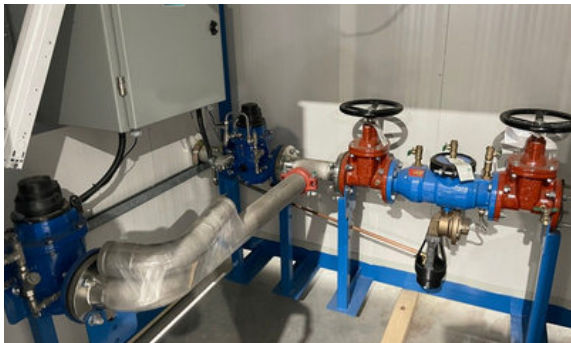
Above: Backflow preventers, actuated slow close control valves, stainless steel piping and Allen Bradley controls provide quality and easy maintenance for years to come.
