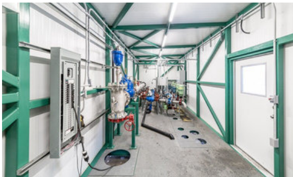
Below: Custom large booster pump station for water dispensing
