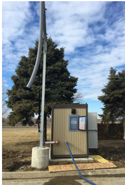
Dual fill (2" upper fill and 3/4" garden hose thread) with custom built self draining fill pipe
