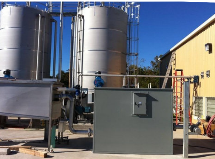
Above: Fats, Oils and Grease acceptance station with separation tank
