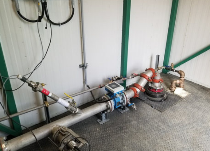
Above: Inline instrumentation to monitor sensitive system parameters. Information about waste is recorded to customer's account.
